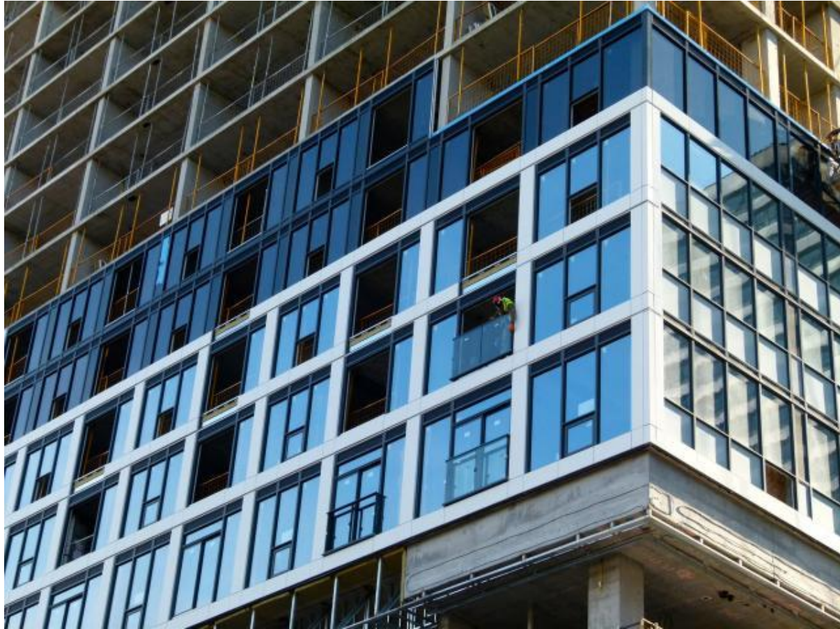
Juliet balconies being installed at Grid Condos, image by Forum contributor skycandy
