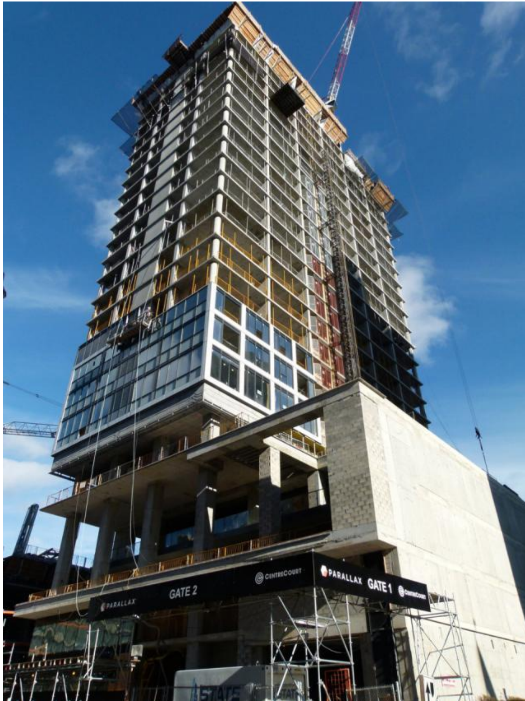
Grid Condos rising above the southeast corner of Jarvis and Dundas, image by Forum contributor skycandy
